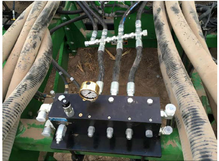
Photo M. Manifold installed on a 60-ft drill with TBT cart. 3 cartridges used, so 3 short feeder hoses going into 4 long 222" feeders, with places for 2 accumulators to plumb into the ends of equalizer fittings.
