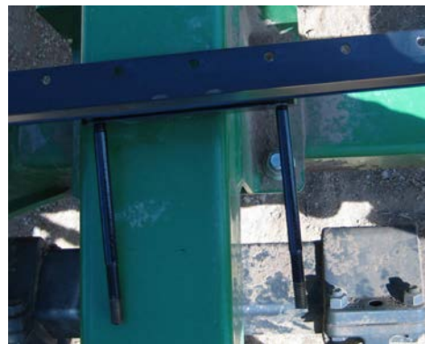
Photo E. RH wing: front, outer end. Brkt #0004 on this 1890. Tray is attached via 1/2 x 3/4" buttonhead bolts threaded into U-bracket. Assembly pulled up off the frame tube for viewing.
