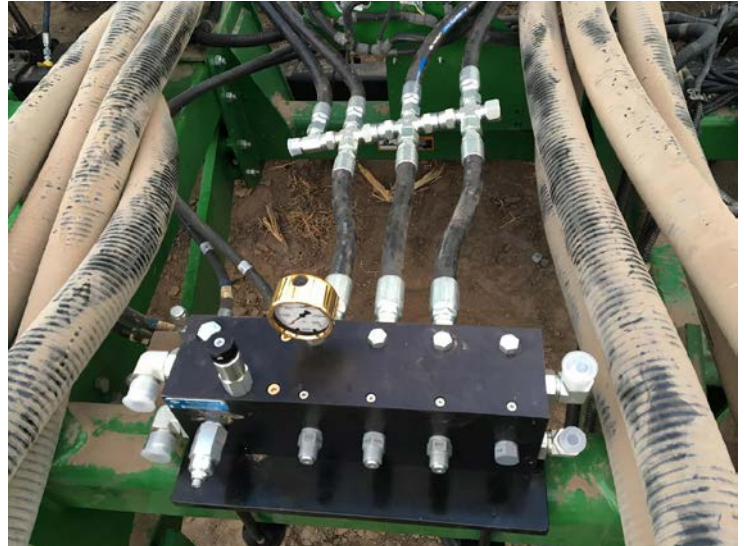
Photo M. Manifold installed on a 60-ft drill with TBT cart. 3 cartridges used, so 3 short feeder hoses going into 4 long 222" feeders, with places for 2 accumulators to plumb into the ends of equalizer fittings.
